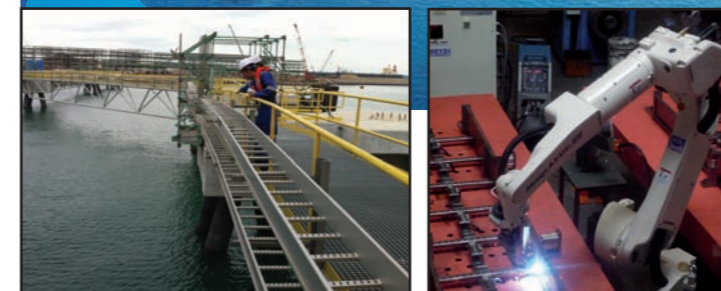
M*RAK cable ladders installed at one of the jetties at SLNG. Welding robot for efficiency and quality consistency
